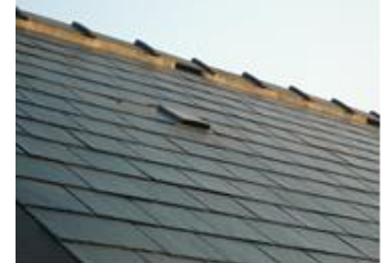
Artificial bat access and roosting compensatory features built into a newly converted barn
