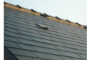
Artificial bat access and roosting compensatory features built into a newly converted barn
